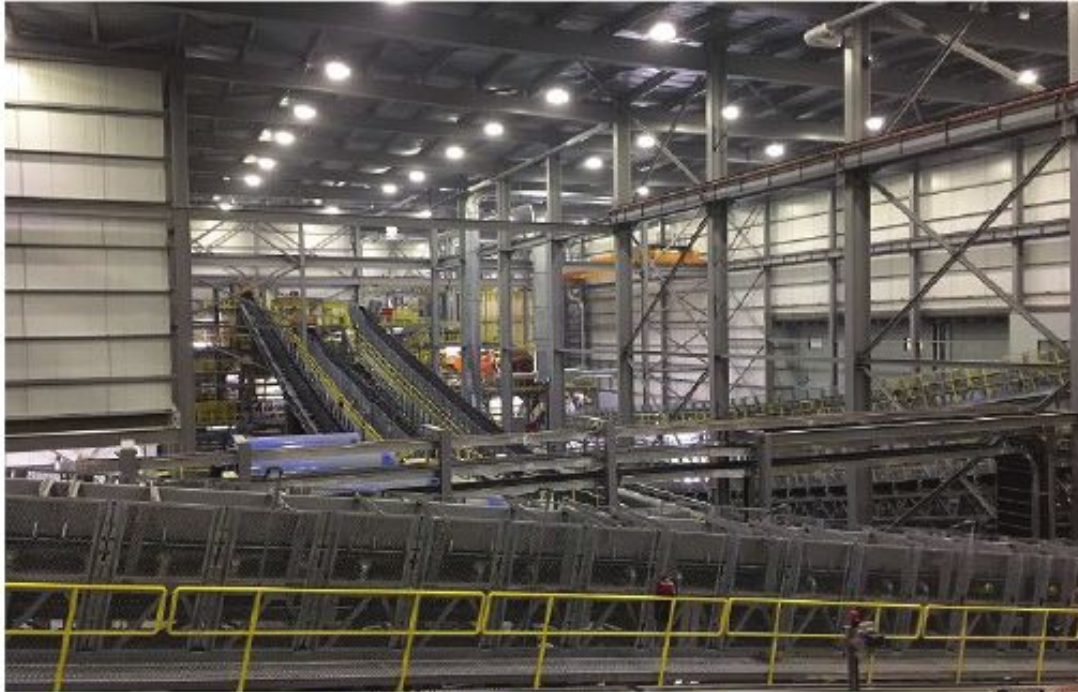
Exhibit 4: Renard processing plant
